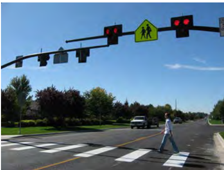
Overhead bike/ped crossing signal
