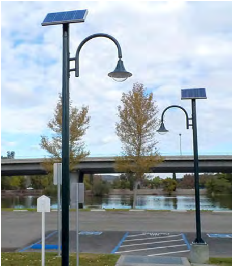
Solar powered pedestrian lights
