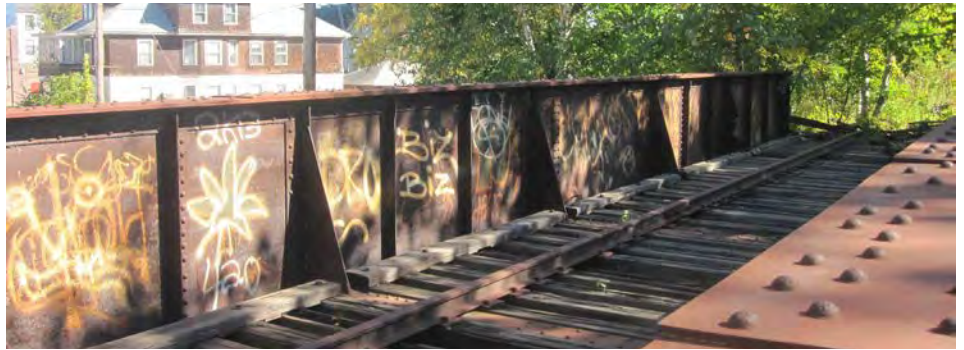
Existing Manchester Street Bridge deck condition
